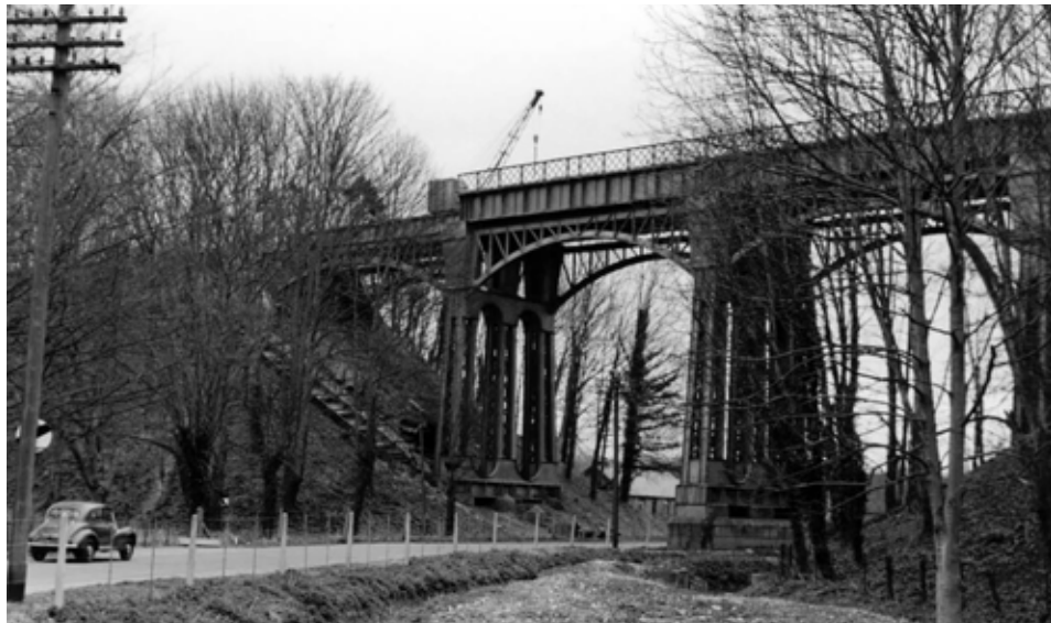
West Meon Viaduct being dismantled March 1957. Photo: Newton Abbot Railway Studies Collection
